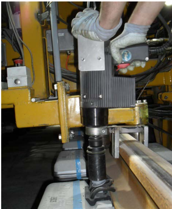
Figure 2: Der alkitronic ® EFCip in operation - Photo: © Alp Transit Gotthard AG
