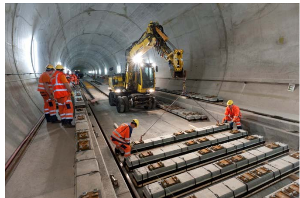
Figure 1: Track construction work in the Gotthard base tunnel – Photo: © Alp Transit Gotthard AG
